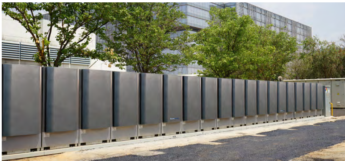
FIGURE 2.6 Commercial fuel cell installation in India
